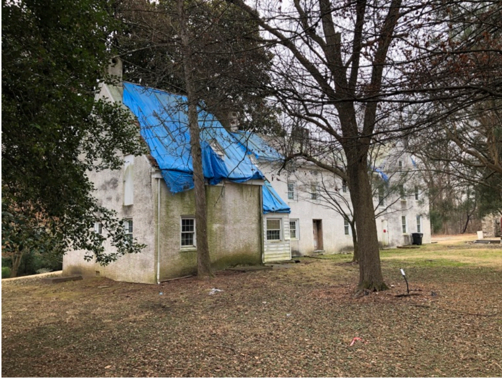
Fig. 34. The north and east side of the house, looking southwest. On the left is the 1946 east side addition to the servants quarters, with the connector just visible with siding. Current photo.
