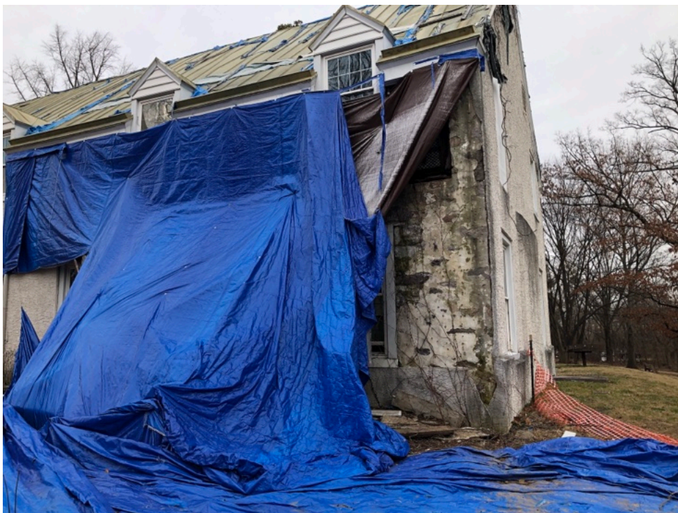
Fig. 49. The southwest corner of the 1932 Okie addition showing the falling away of the stucco on mesh, revealing the intact original stucco on stone.
