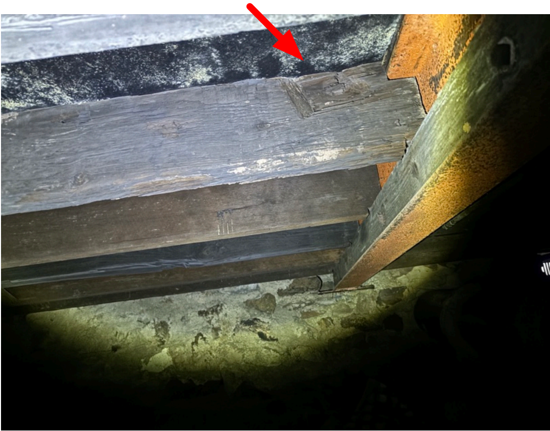
Fig. 33. Joist under the house east of the circa 1810 addition, showing a cut possibly made by hand tools. From the archive of the King of Prussia Historical Society.
