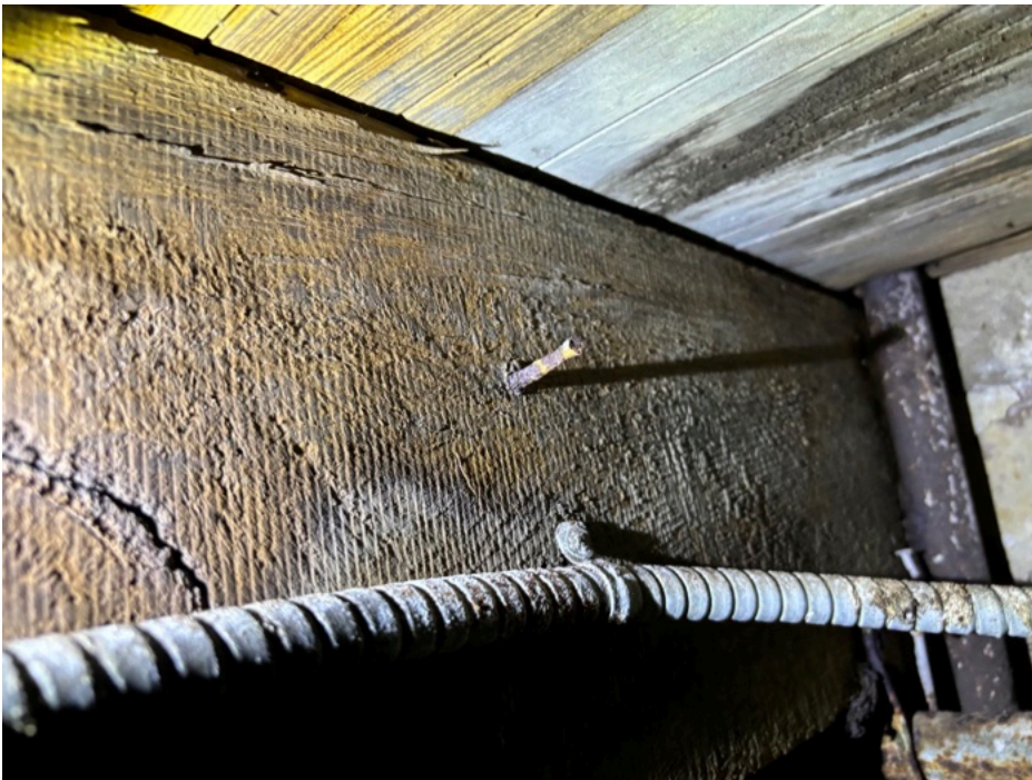
Fig. 24. Joist under the circa 1810 stone addition showing vertical, evenly spaced saw marks. From the archive of the King of Prussia Historical Society.
