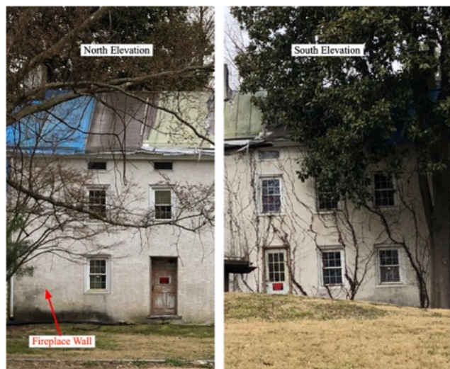
Fig. 20. North and south elevations of the c. 1810 portion of house, annotated. Created from current photos.
