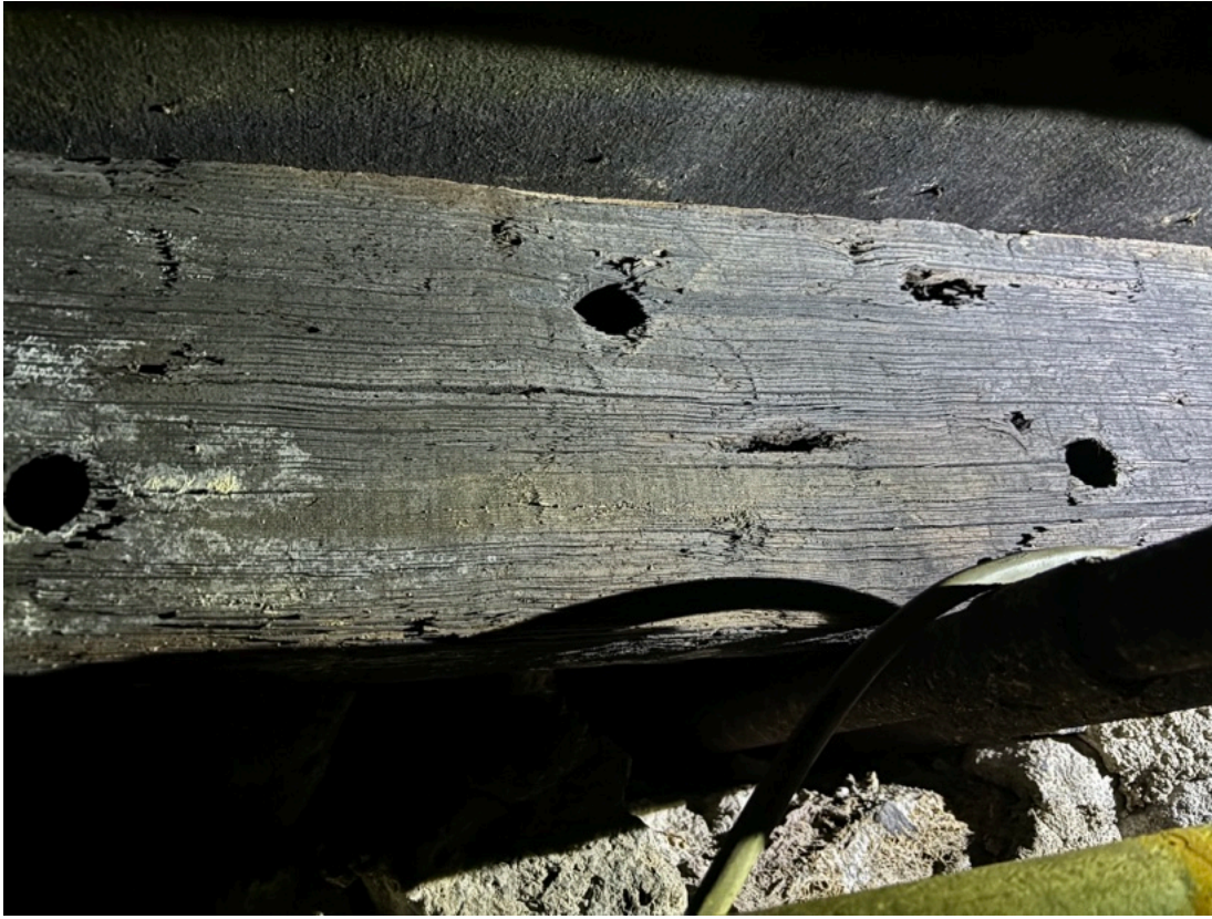
Fig. 31. Joist under the house east of the circa 1810 addition, showing marks not indicative of machine sawing. The holes may have been for wood dowels, which were often used before iron nails became available in large quantities. From the archive of the King of Prussia Historical Society.
