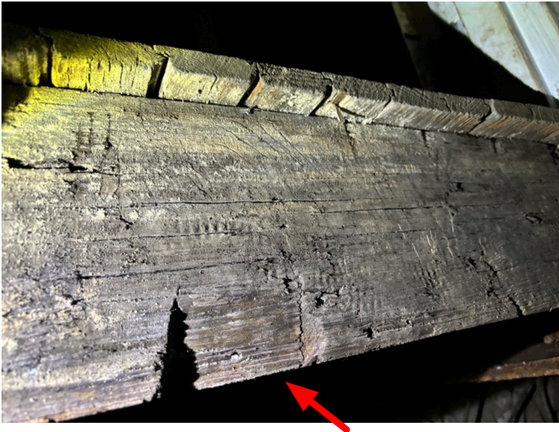
Fig. 32. Joist under the house east of the circa 1810 addition, showing a cut possibly made by hand tools. From the archive of the King of Prussia Historical Society.
