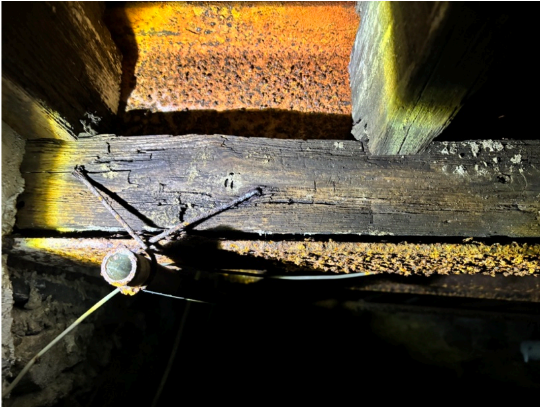
Fig. 29. Joist under the house east of the circa 1810 addition, showing marks not indicative of machine sawing. From the archive of the King of Prussia Historical Society.
